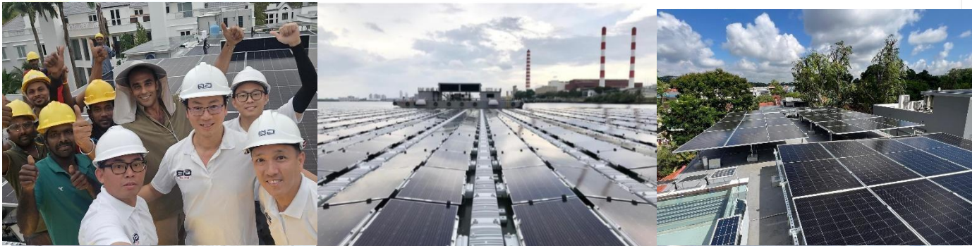
Design Integration & Engineering Excellence Solar Energy Systems to the environment
